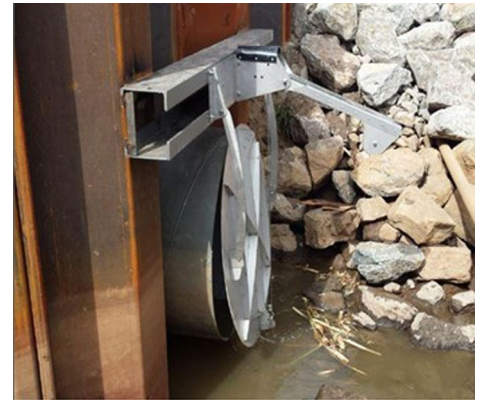
Adding a simple fish portal like this one next to the Palo Alto Tide Gate could help steelhead trout return and flourish in our city. Photo: S. Scott & Associates. https://ssaenvironmental.com/fish-friendly-tide-gates/
