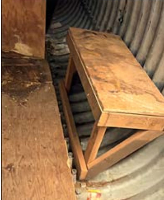
C - This shot shows the underground living area in a corrugated steel pipe about five or six feet in diameter, with a flat wooden floor to facilitate walking and a bench to sit on. The view is to the south (toward the street). The half-partition, presumably for privacy, blocks the view of the south part of the shelter, which holds a short, narrow sleeping bench.
