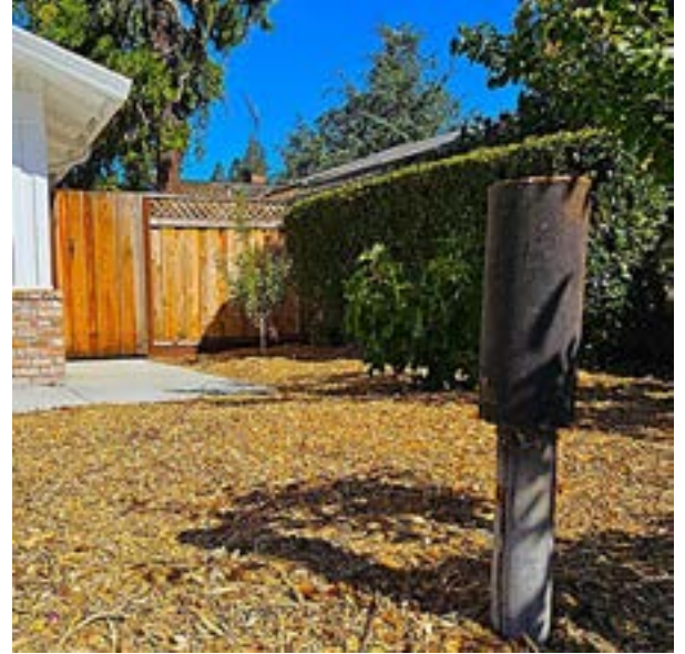
E - The vent sticks up about 18 inches above ground level and has a rain cap to keep rainwater from entering the shelter. It is in the front yard near the driveway and street.
