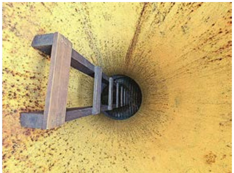
B – The ladder. This shot is straight down into the rusty pipe, about seven feet to the bottom. The wooden ladder is firmly fixed to the pipe and shows no rot or damage.
