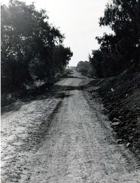
Illustration 17: The torn-up bike path, used as a haul road in 1996 for the underground bypass flood culvert construction. Photo by Mollie Graham.
