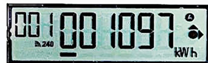
Close up of display on new smart electric meter shows the number of total Kilowatt-hours of energy used by the customer.
