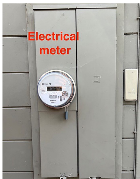
This unit includes a smart electric meter on the left; the main electric service panel is under the cover on the right.
