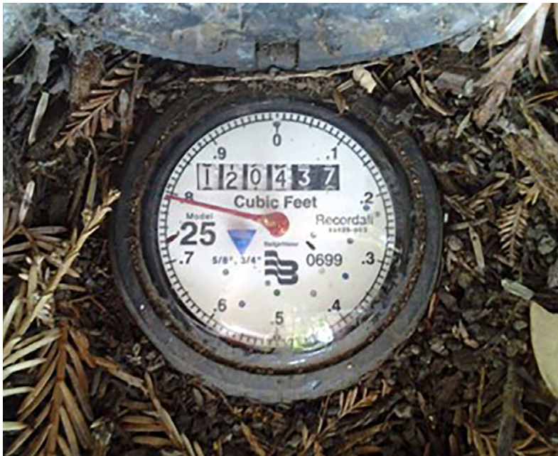
Water meter photo #1. Photos by David Coale
