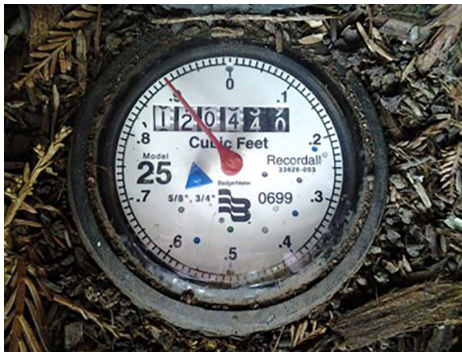
Water meter photo #2.
