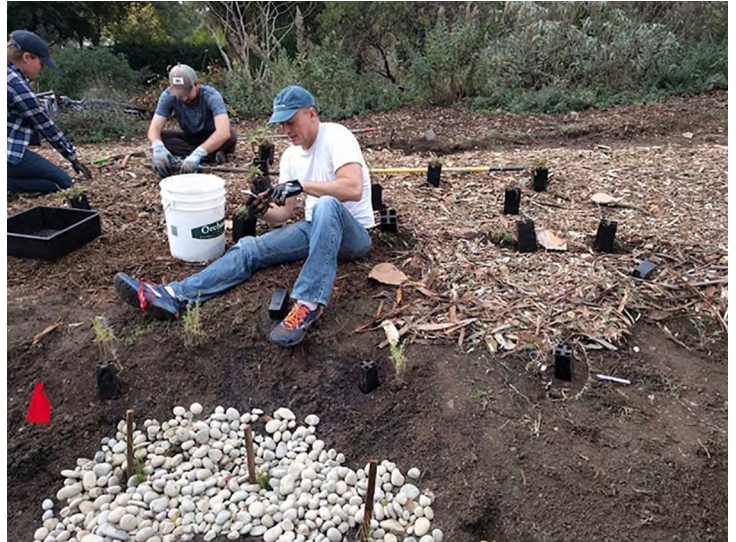
Fall 2018: Volunteers installing the Rain Garden at the Bol Park Native Garden.
