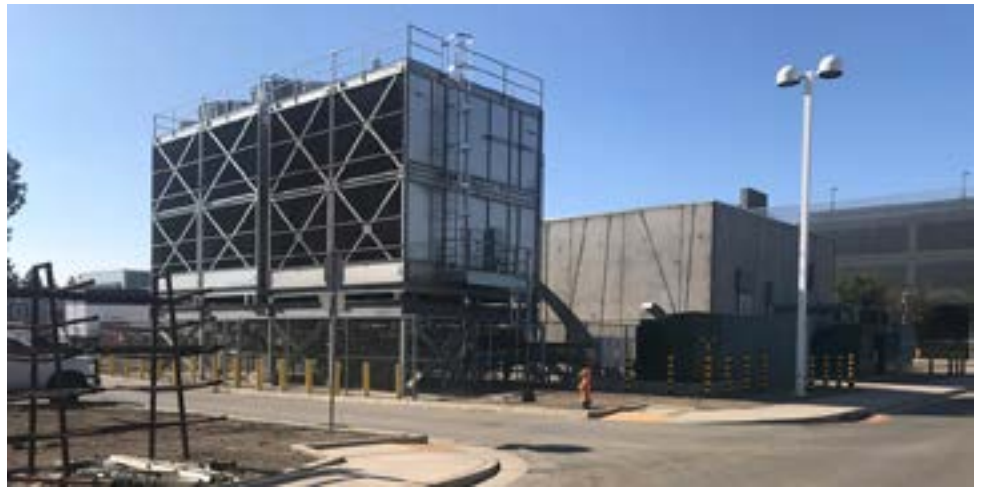
The VA Hospital cooling tower near Barron Park. Photo: Justin Kitch
